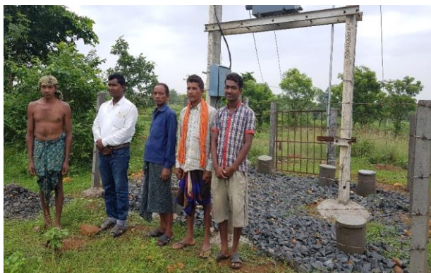
Electric transformer and 7 HP pump in power house installed by OAIC in Dudhiasole village
