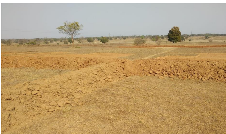
Initiation of field bunding and land levelling on barren land in Barbil village
