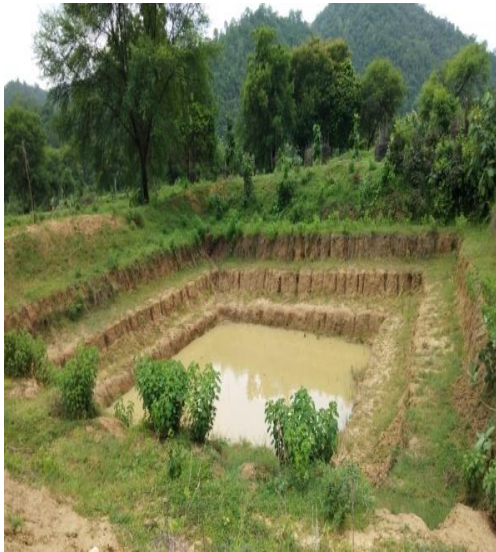
Farm pond constructed in command area on land of Champeswar Hans with support from Horticulture Department
